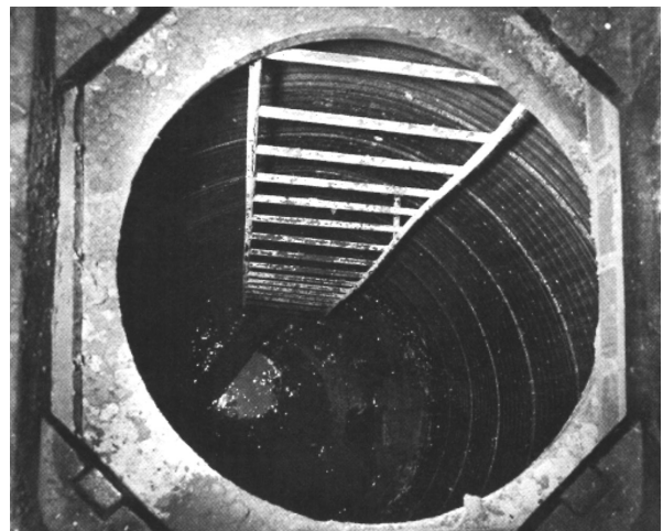
Ladder Mounted on Riser.
